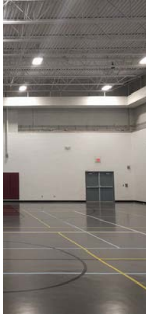
Converted all municipal building lighting to LED (GAT 14)
