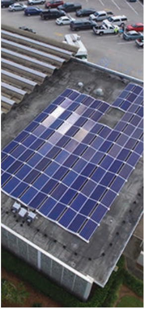
Installed an 83 kW Solar PV System on City Hall (GAT 1)
